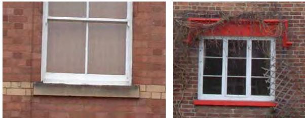
Stone cills (above) were common in the mid-late 19th century, although many are now painted.
