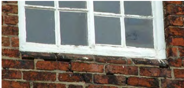
Above - where there was no cill, as with many of the smaller cottages and the less important elevations of the town houses, the window joinery was positioned close to the face of the wall. In the example above handmade bricks were moulded to create a weathering.
