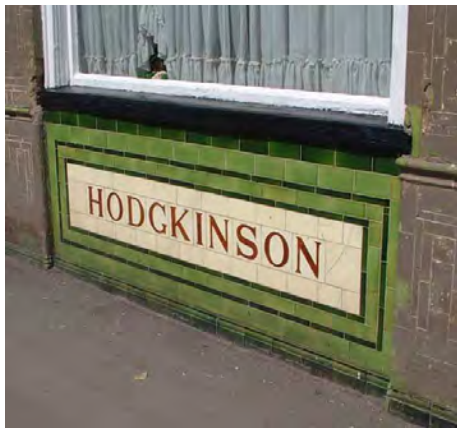
Below - tiled stall risers at 46 High Street (formerly Hodgkinsons butchers) and 5 Derby Road (bottom).
