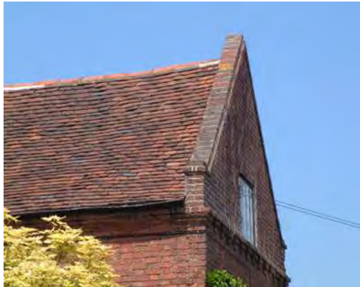
Above - raised coped brick gable. These were generally used on the higher status buildings during the mid-late 18th century.
