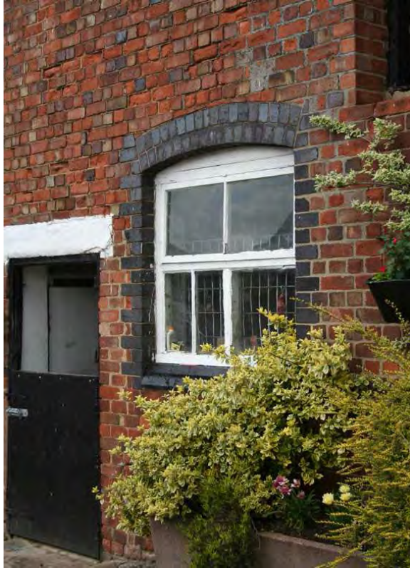
Above left - segmental blue brick arch, with blue brick reveals and moulded brick cill at The Creamery.
