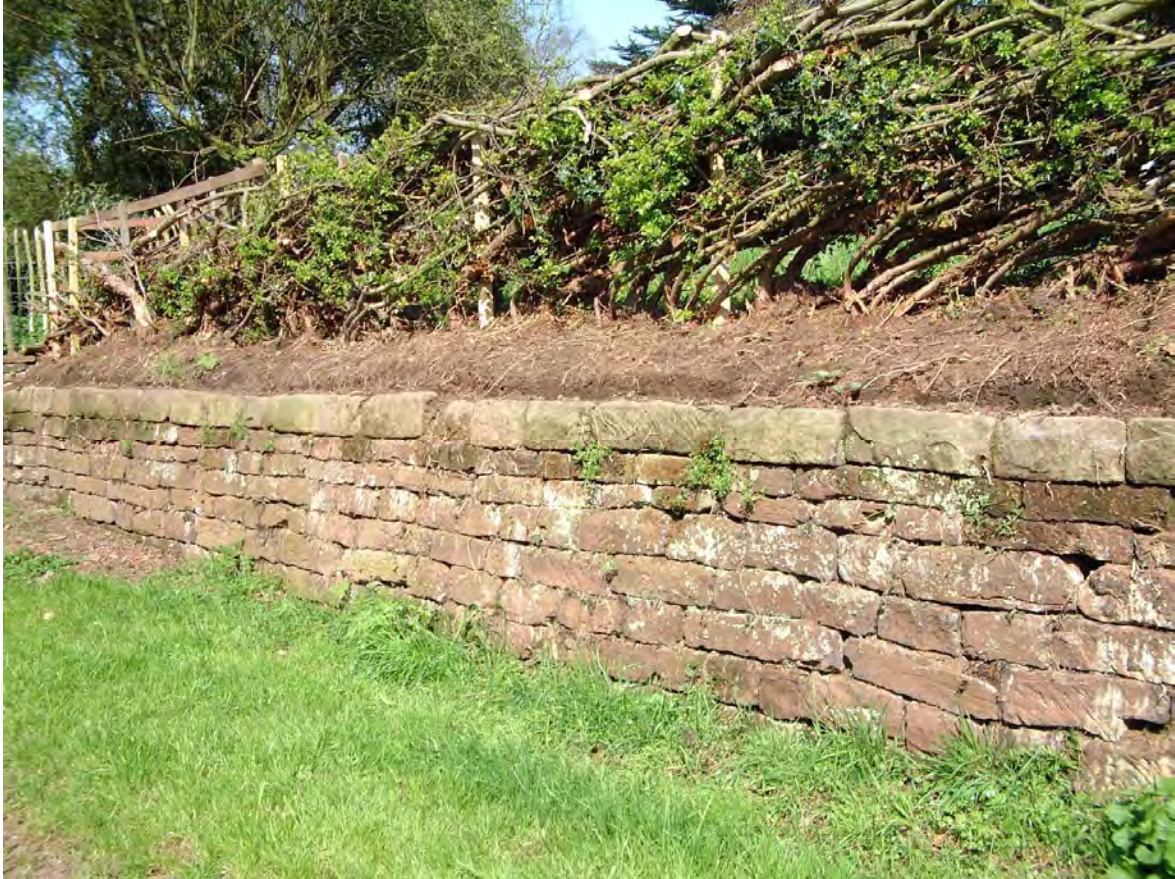
Many of the walls around the Newton Park estate were built in an evenly coursed pinkish sandstone (as at Farm Lane - above).
