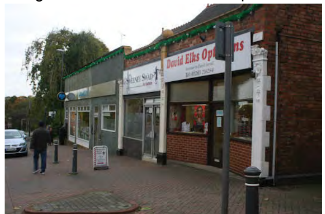
Midland Road - loss of terracotta parapet and pilaster details
