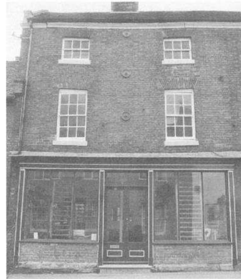
Rebuilding the front of this Grade II Listed Building has been avoided by using steel supports and straps which are largely concealed
